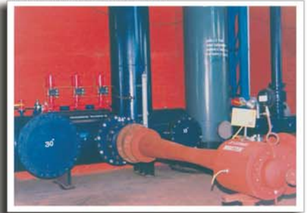
Main discharge header has three connections for testing ejectors on different diameter lines.
