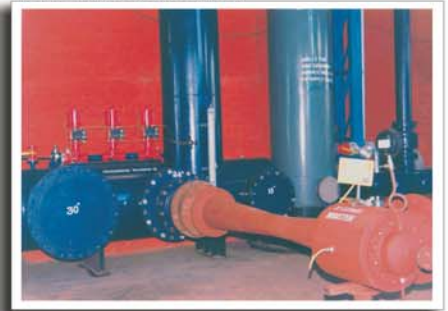
Main discharge header has three connections for testing ejectors on different diameter lines.
